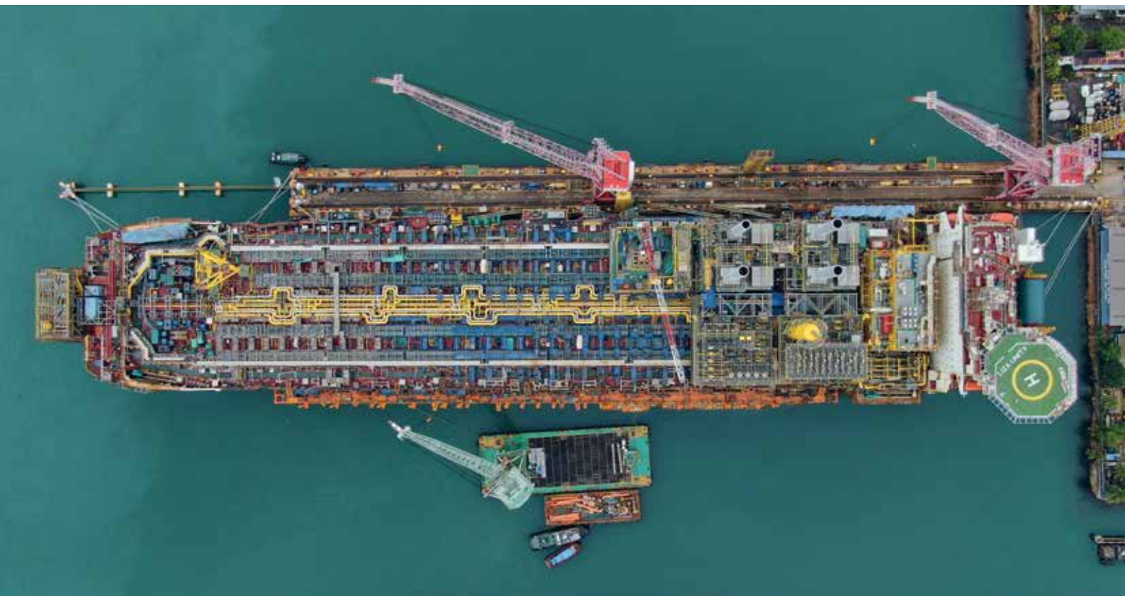
The topsides lifting campaign for the Liza Unity FPSO was completed in March 2021 with over 26,000 tons of topsides lifted in position
